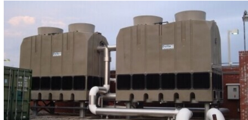
Example wet water cooling towers
